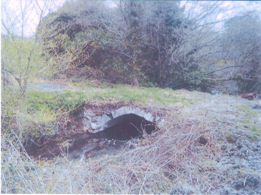
Very flat arch and missing keystone
